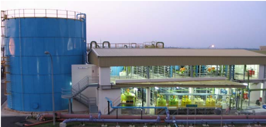
Figure 2: Senoko Desalination Plant, commissioned in 2004, makes use of triple membrane technology to provide ultra-pure product water that requires little further water treatment for boiler feedwater boiler.
