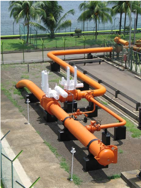
Senoko Pig Receiving Facility (SPRF)
